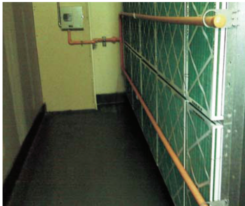
The VESDA by Xtralis air-sampling pipe network does not interfere with the fan filters or ongoing maintenance at the Wells Fargo Center in Minneapolis.
