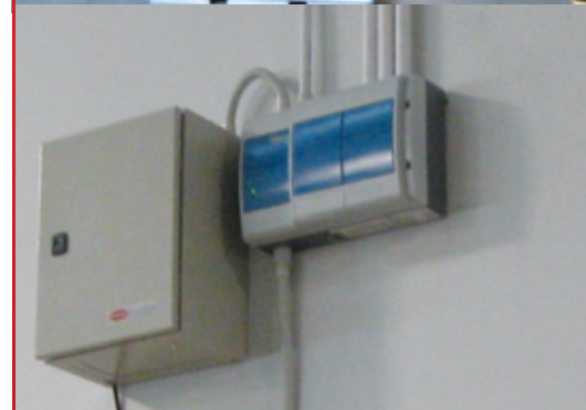
Direct connection from the VESDA detector to the existing security panel met the insurer's requirements.
