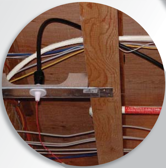
Sampling pipes can be hidden in roof spaces so that the only visible component is the tiny sampling point.
