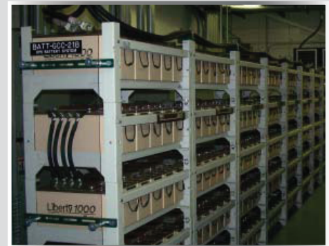
A data center in the Midwestern United States is using VESDA ECO for hydrogen detection in three battery rooms.
